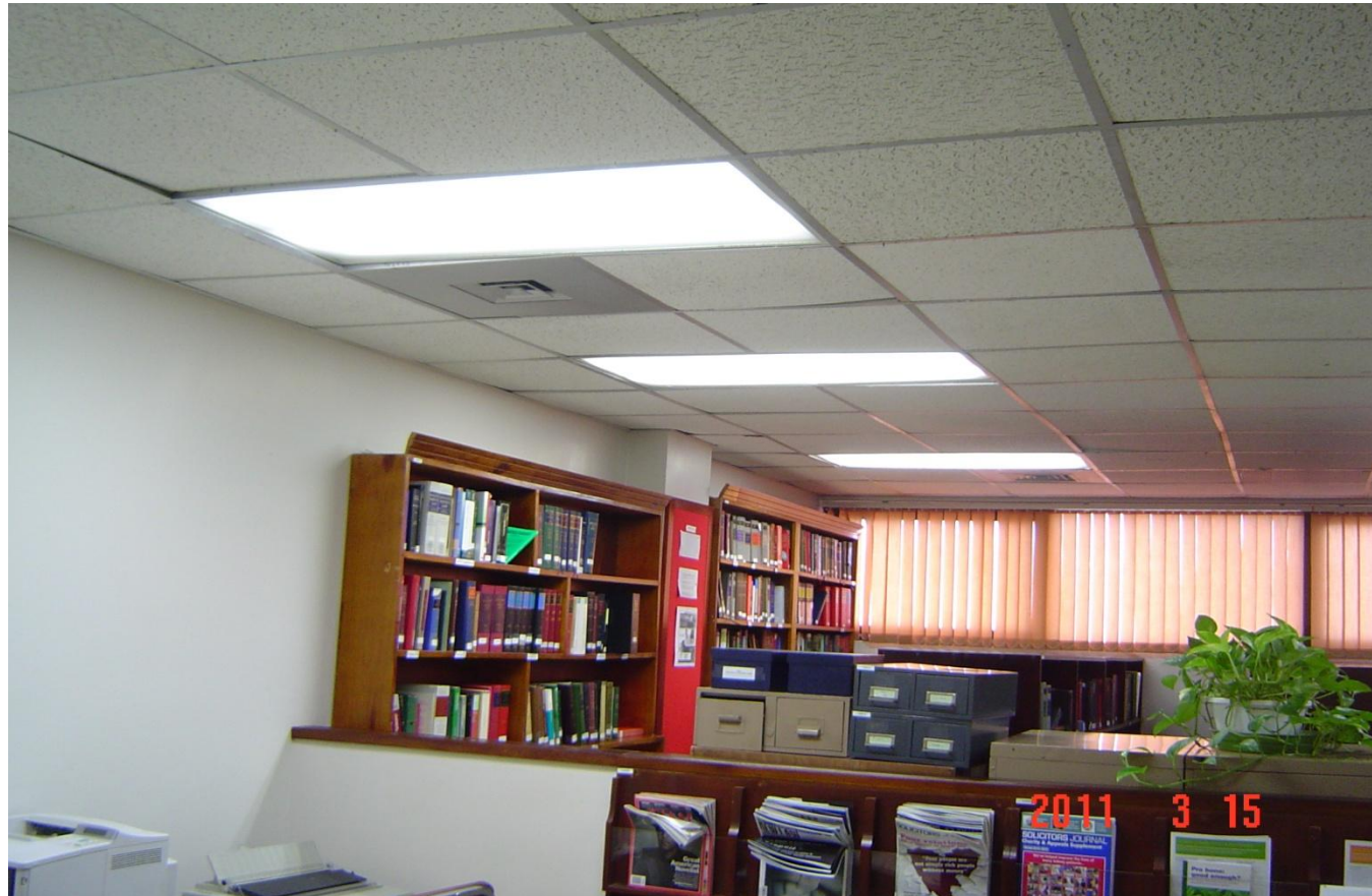
LED Lighting Installations at Dunn Cox & Associates
